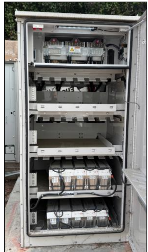
Battery Backup for a Macro Site
