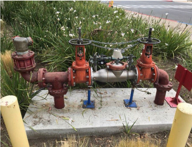
3 - FIRE PROTECTION BACKFLOW PREVENTER
