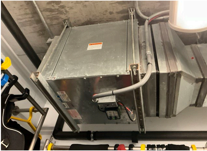
13 – VARIABLE AIR VOLUME UNIT
