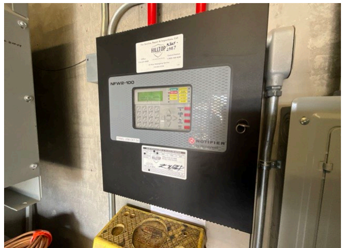
16 – FIRE ALARM PANEL
