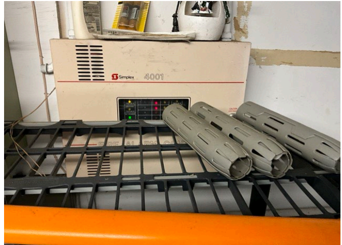
18 – FIRE ALARM PANEL
