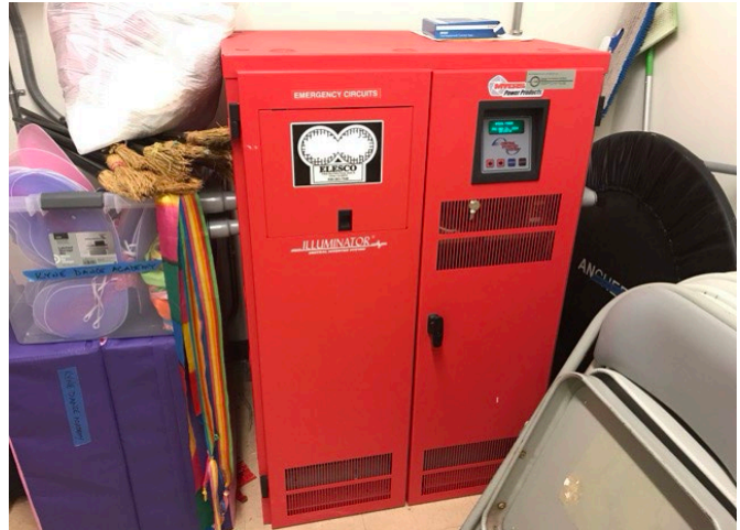
30 – UNINTERRUPTIBLE POWER SUPPLY
