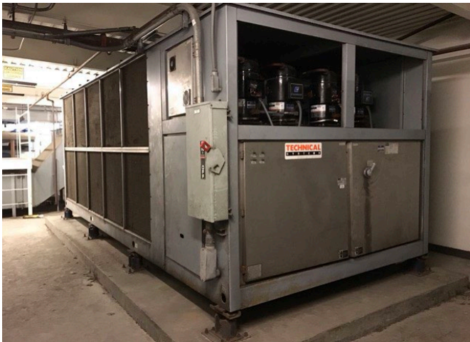
23 – AIR CONDITIONING UNIT
