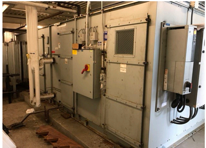
22 – AIR HANDLER UNIT
