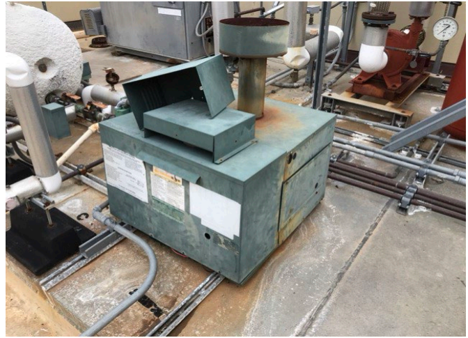
26 – DOMESTIC WATER BOILER
