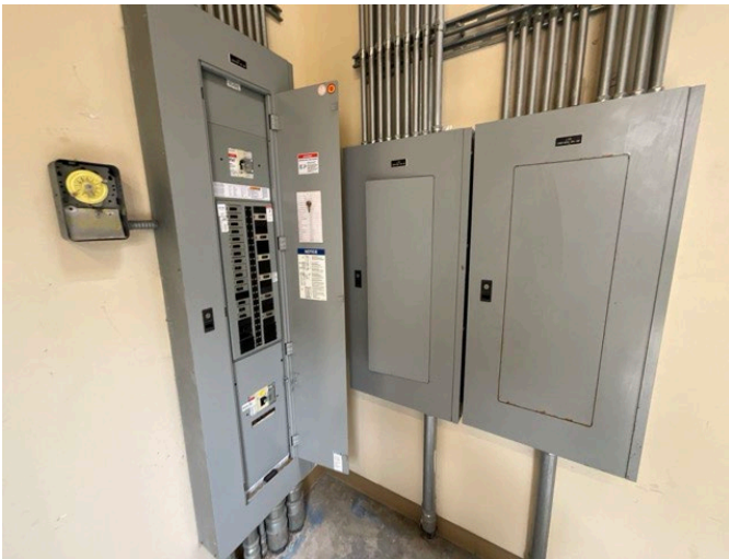
13 - MAIN DISTRIBUTION PANEL
