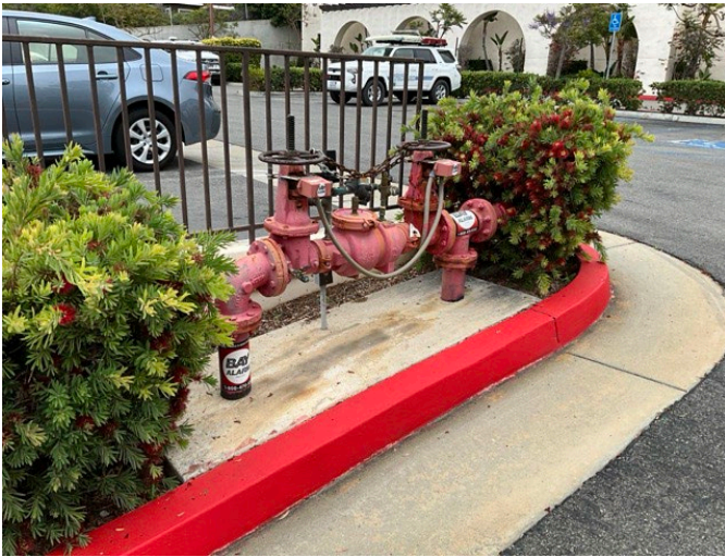
3 - FIRE BACKFLOW PREVENTER
