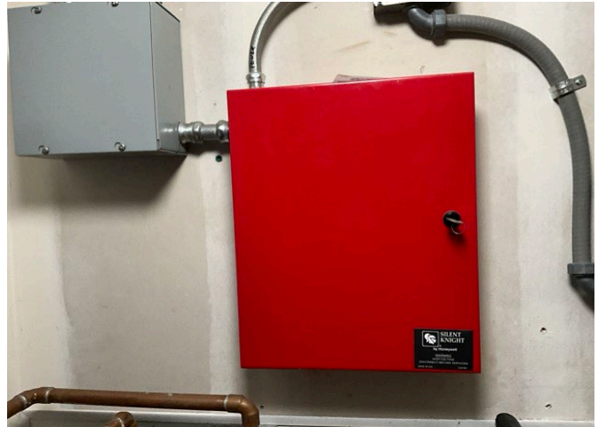
18 – FIRE ALARM PANEL
