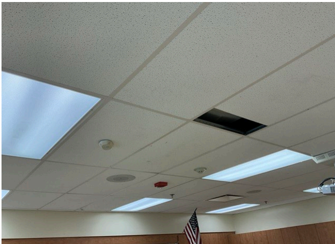
17 – FIRE ALARM SYSTEM COMPONENTS
