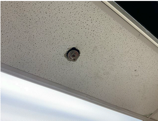
13 - FIRE SUPPRESSION SYSTEM
