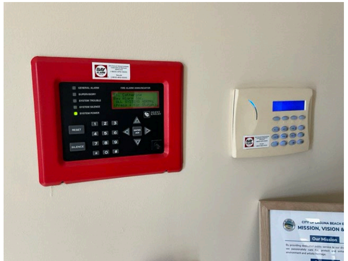
14 - FIRE ALARM PANEL
