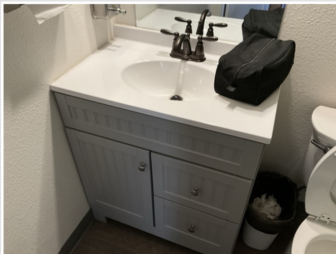
LAVATORY WITH NO CLEARANCE
