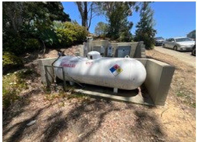
6 – SITE PROPANE AND ELECTRICAL
