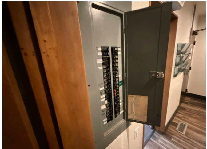
18 – MAIN DISTRIBUTION PANEL
