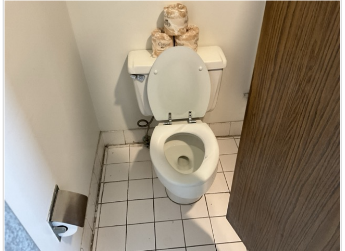
TOILET STALL NOT ACCESSIBLE
