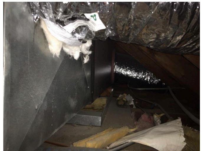
22 - AIR HANDLER UNIT
