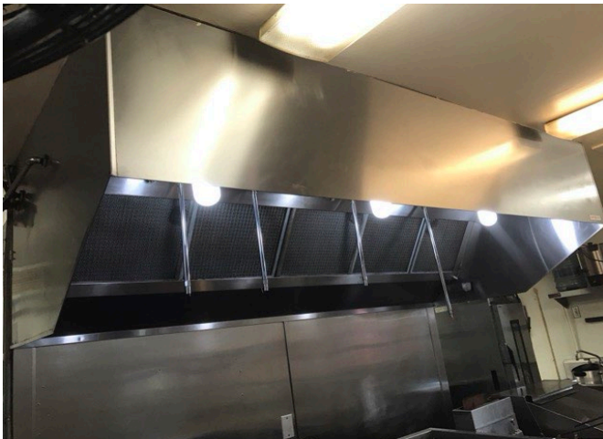
17 – FOODSERVICE EXHAUST HOOD
