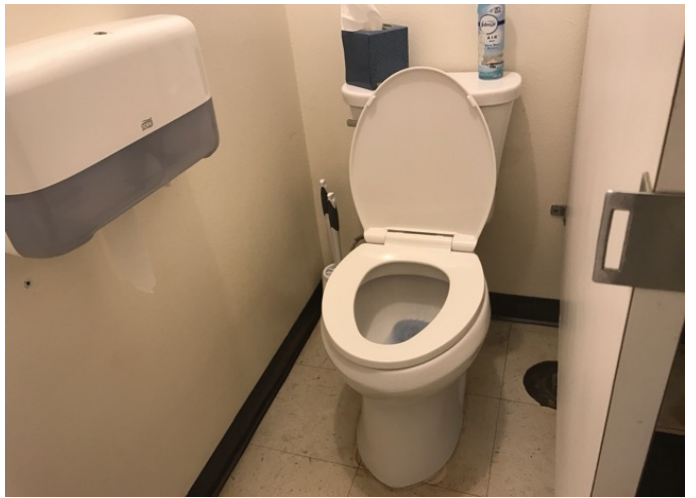
IRVINE BOWL BACKSTAGE TOILET AND STALL NOT ACCESSIBLE
