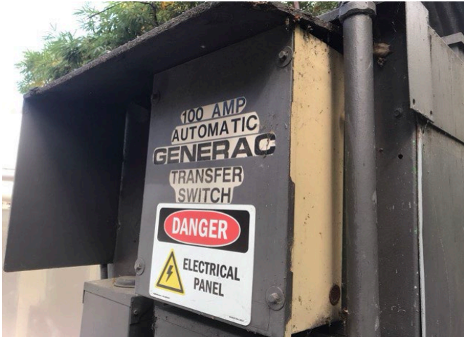
11 – AUTOMATIC TRANSFER SWITCH
