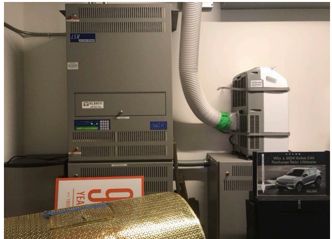
10 – UNINTERRUPTIBLE POWER SUPPLY
