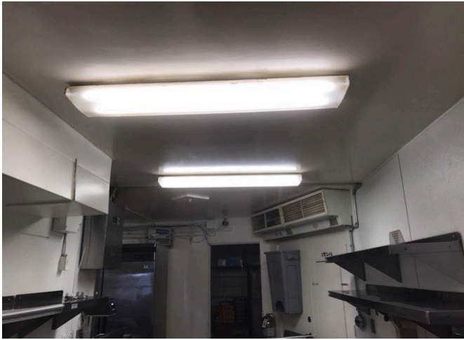
19 – INTERIOR LIGHTING SYSTEM
