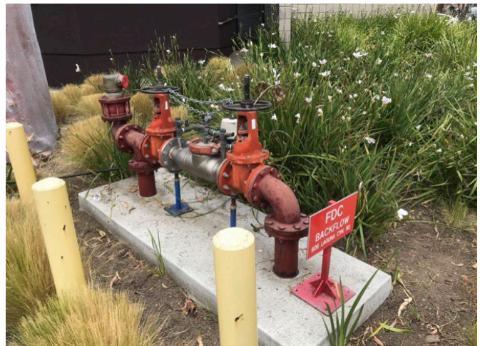
6 – FIRE PROTECTION BACKFLOW PREVE
