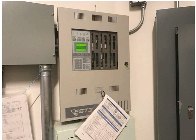
12 – FIRE ALARM PANEL
