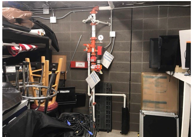
12 – FIRE SUPPRESSION SYSTEM
