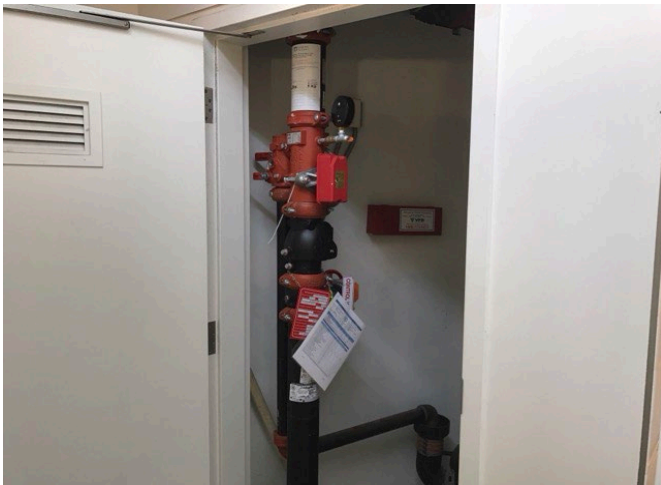
9 – FIRE SUPPRESSION SYSTEM
