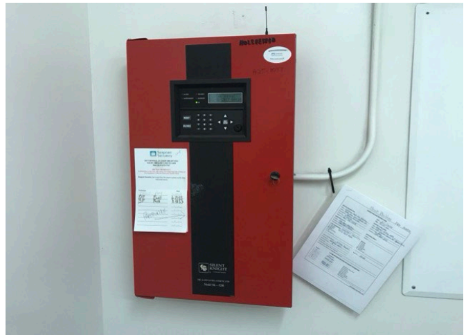
10 – FIRE ALARM PANEL
