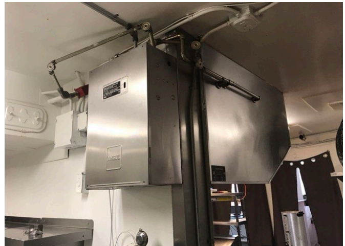
18 – FOODSERVICE FIRE SUPPRESSION S
