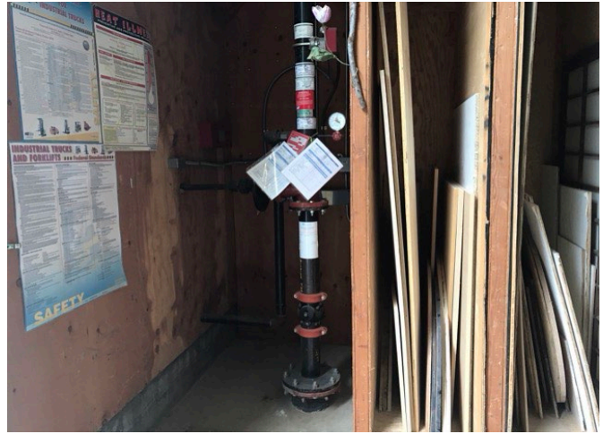
8 – FIRE SUPPRESSION SYSTEM
