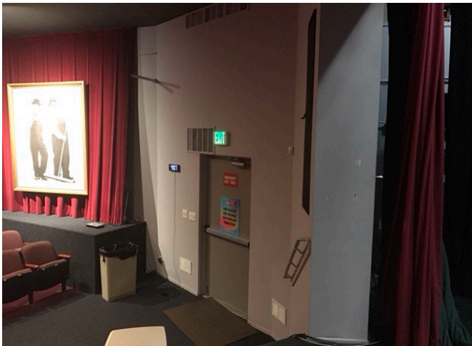
21 – FIRE ALARM SYSTEM
