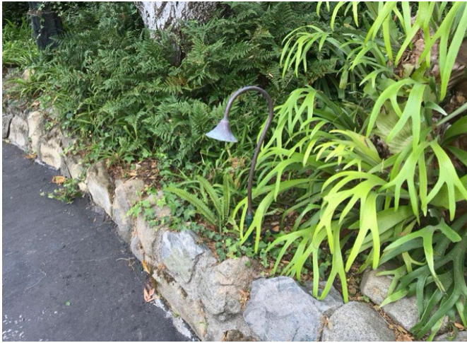
7 – SITE WALKWAY FIXTURE W/ LAMP
