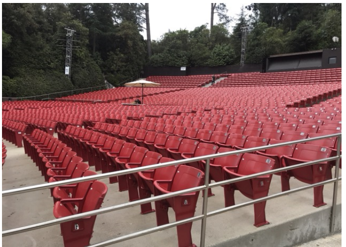
IRVINE BOWL ACCESS TO SEATS ABOVE ACCESSIBLE SEATING ROW REQUIRE STEPS
