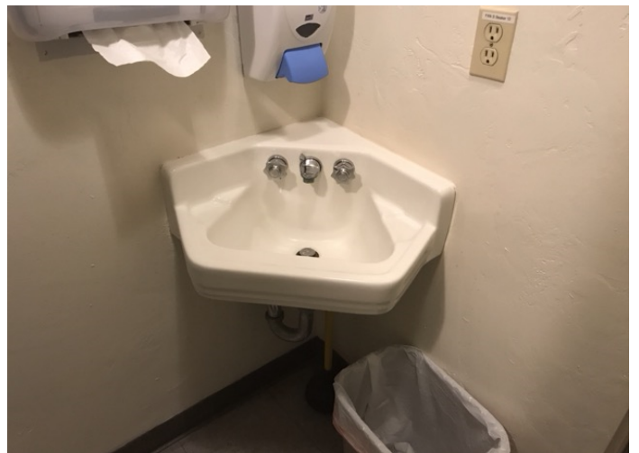
FORUM BACKSTAGE SINK HANDLES NOT ADA COMPLIANT
