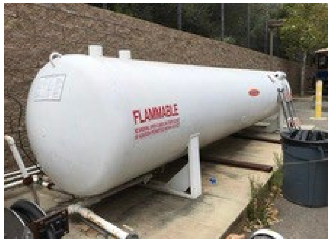
10 – ABOVE GROUND FUEL TANKS
