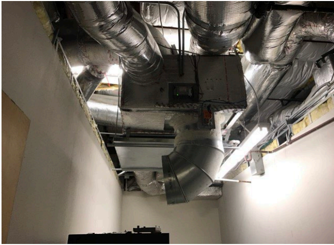
19 – SPLIT SYSTEM AIR HANDLER
