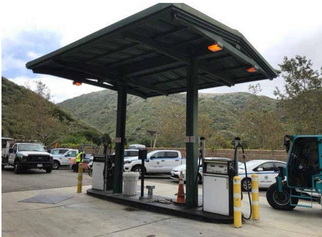
9 – FUEL PUMPS AND CANOPY
