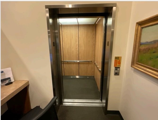
LOBBY LOOKING AT CABS (WITH DOORS OPEN)
