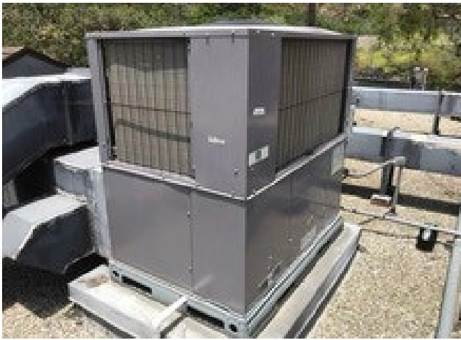
15 – PACKAGE ROOFTOP UNIT
